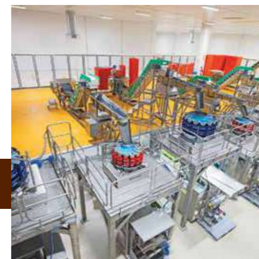
Pattyn Packaging Automation & Palletizing Robots. 6 vertical retail packaging lines, pillow pack, quattro seal, block bottom, ro-pack and Doypack
