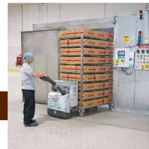
Oven treatment facilities
